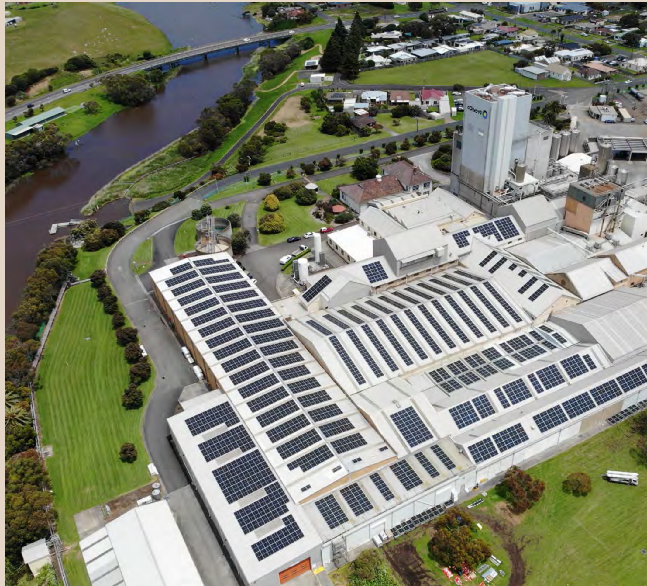
Image of a CIM financed distributed rooftop solar system in Dennington, VIC.
